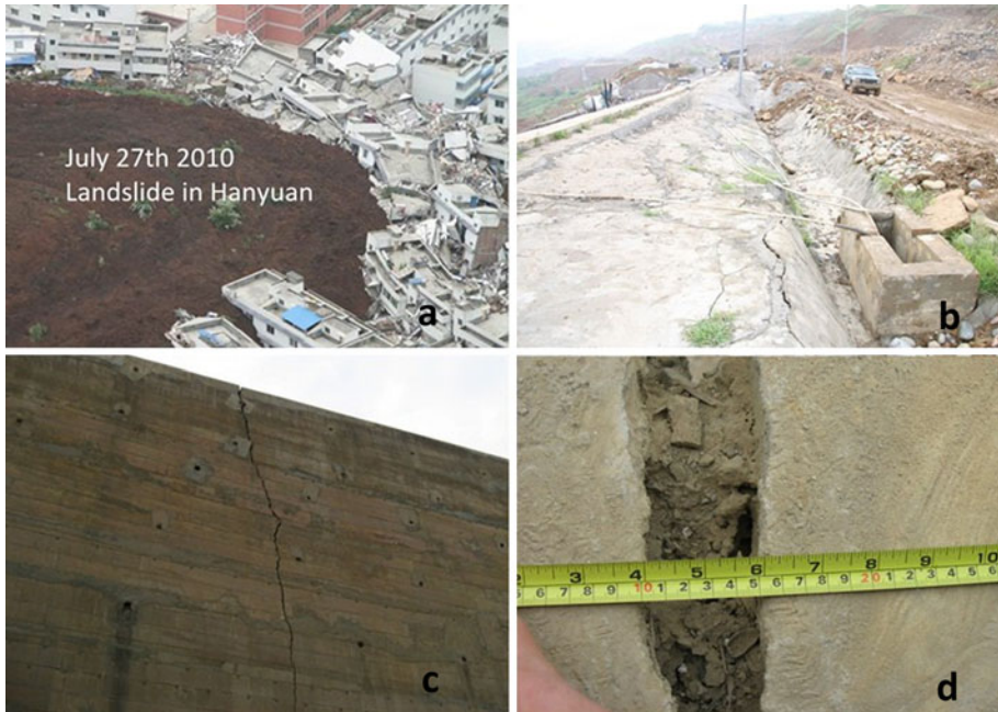
Fig. 2 Landslide failure in 2010 and cracks observed on the retaining walls
