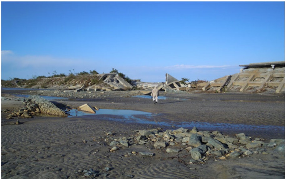
Fig. 5 Extensive failure due to overtopping of coastal dikes in Soma City, Fukushima Prefecture. The parts of the structure that survived had armour units placed in front of them
