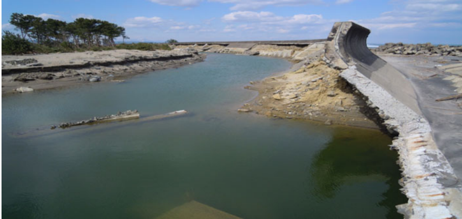
Fig. 6 Failure of coastal dikes in Watari. Note how scouring of the back of the dike can then result in the exposure of the core soil, which can then lead to the failure of the unsupported concrete superstructure of the dike
