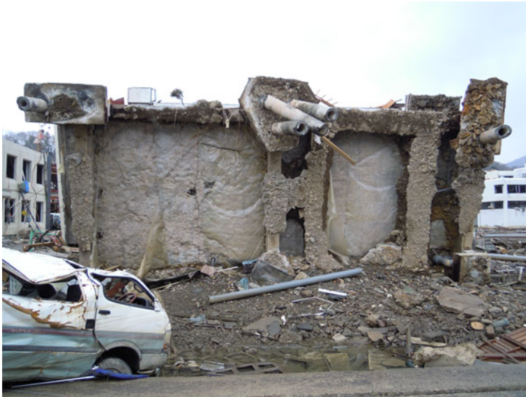
Fig. 3 Reinforced concrete building damaged due to overturning in Onagawa. The piles on which the building was anchored failed in shear
