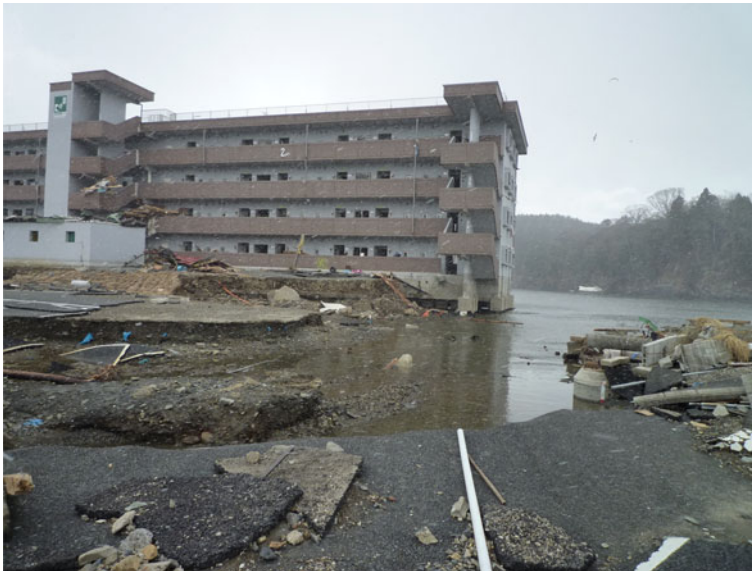
Fig. 2 Surviving Evacuation Building in Minamisanriku. The tsunami inundation reached the top of the building. Generally, the building was well constructed and suffered little structural damage, aside from scouring at the sides
