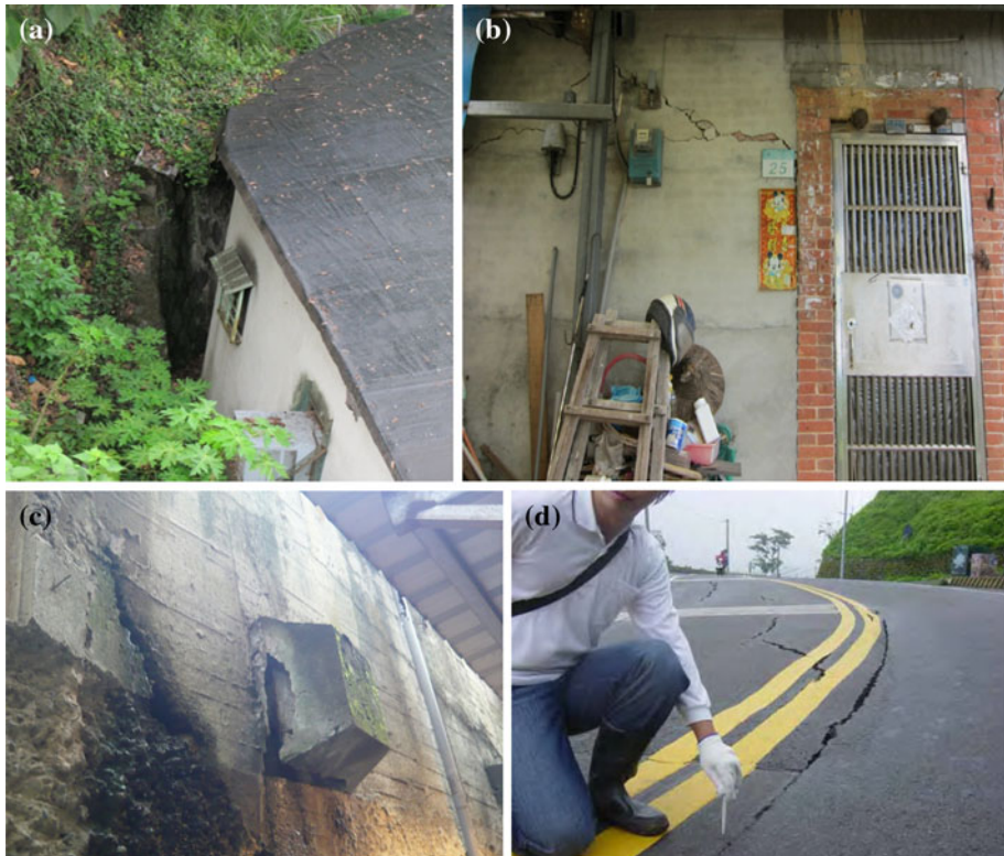
Fig. 6 Photographs indicating landslide potentials: a buildings have insufficient distance from retaining structures; b cracked walls; c ground anchor is cracking and peeling; d nearby roads have cracks
