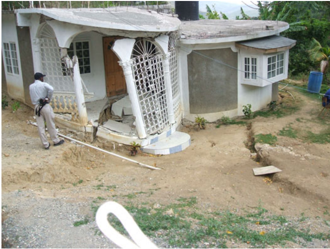
Fig. 5 A private home built in southeast St. Andrew, Jamaica is severely damaged by a rainfall-triggered landslide. Differential movement on parts of the landslide has produced cracking in the foundation and adjacent structural elements. The underlying bedrock in this area consists of shale and mudstone of the Lower Eocene Richmond Formation, which was shown by Ahmad and McCalpin (1999) to be susceptible to deep landsliding
