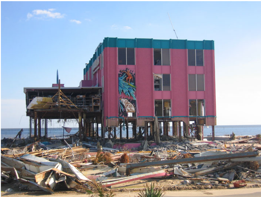
Fig. 1 Casino in Biloxi, Mississippi, USA after Hurricane Katrina in 2005 (© Munich Re)
