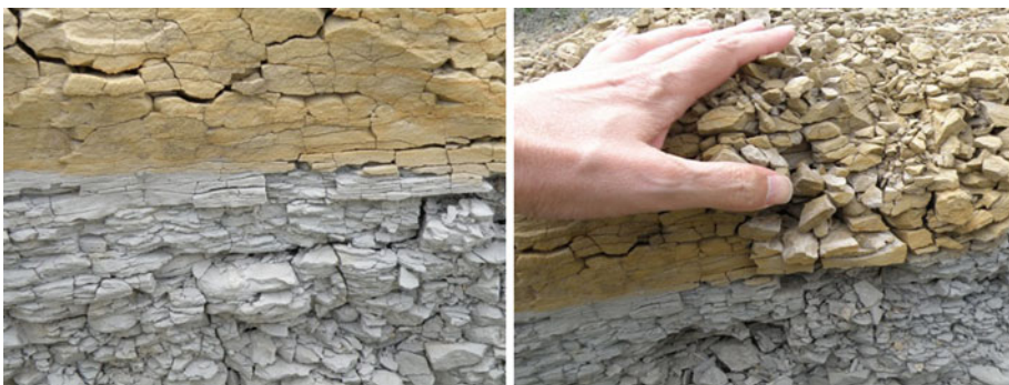
Fig. 2 Weathering and decomposition of flysch rock mass exposed to water and atmospheric conditions
