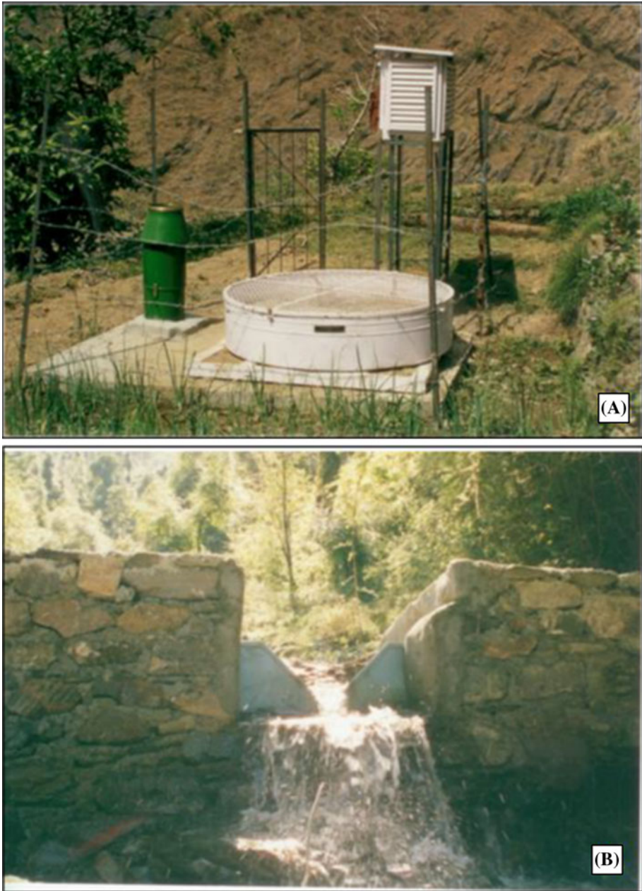
Fig. 3 a Meteorological station installed at high altitude of each sample micro-watershed. b Hydrological station installed at the mouth of each sample micro-watershed
