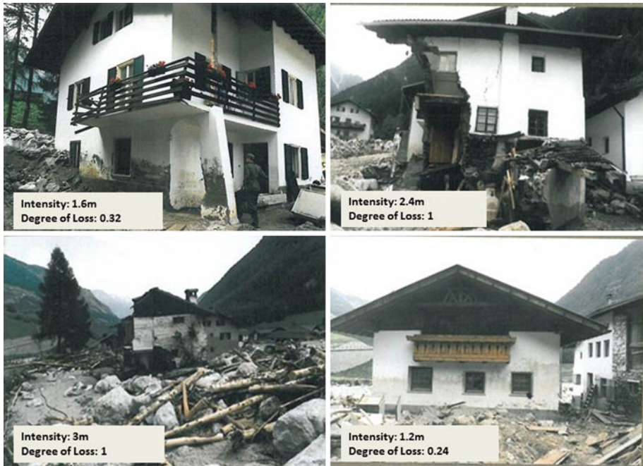
Fig. 3 Photographs of damaged buildings following the event of August 1987 (Source: Municipality of Martell) with assessed intensity as deposit height and the corresponding degree of loss
