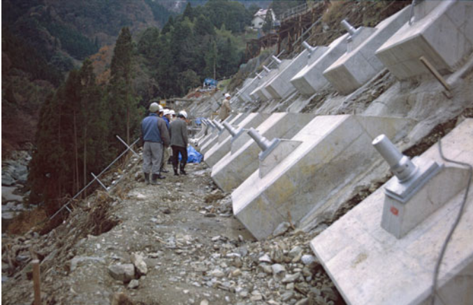
Fig. 8 Stabilisation works at Zentoku landslide on Shikoku Island, Japan. The large concrete blocks are the head units for rock anchors. This type of stabilisation is not only costly, involving drilling and grouting of steel bars, but is also quite time-consuming especially where access is difficult
