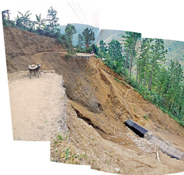
Fig. 5 Landslide on the B1 road at Section in Portland Parish, Jamaica. This event severed much of the local coffee production industry from the ports used to ship the product to market. (This picture is a photo-collage and some distortion is inevitable)
