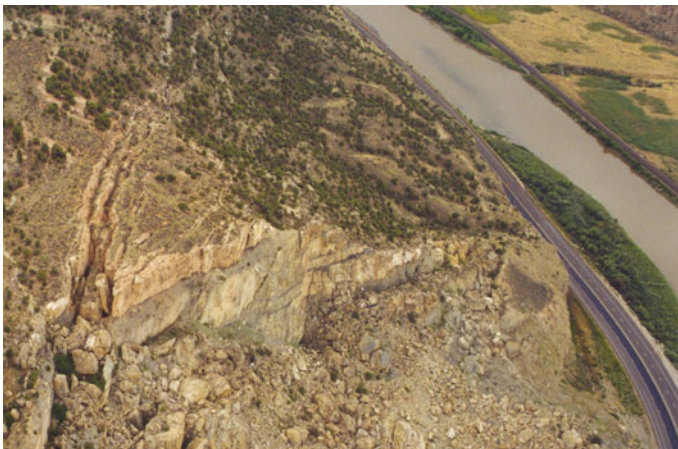
Fig. 6 DeBeque Canyon landslide in Colorado, USA—the photograph is taken from the head of the landslide. Interstate 70 passes over the toe although the original toe extends to the other side of the Colorado River. The proximity of the river and railway are also evident, and a fissure is shown close to the head of the slide on top of which debris is clearly visible. (Image by kind permission of Jonathan L. White, Colorado Geological Survey)
