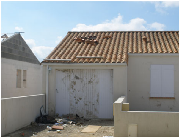
Fig. 5 In La Faute-sur-Mer, rescue services gained access inside the house by lifting roof tiles. (photo: F. Vinet)
