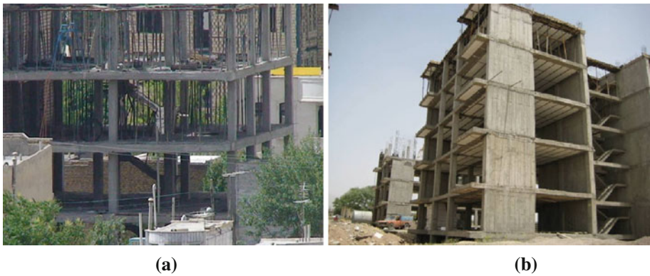
Fig. 4 Samples of RC building types (Derakhshan 2009). a RC moment frames. b RC shear walls
