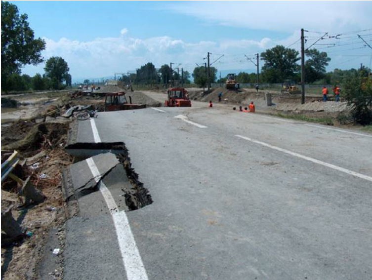
Fig. 14 The destruction of the national road and railway Tecuci-Marasesti (Romanescu 2005)
