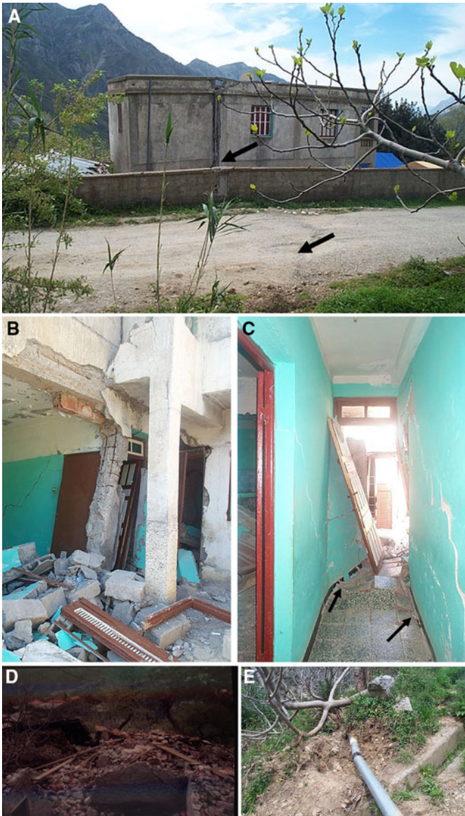
Fig. 10 Effect of the landslide on construction and facilities. a Outside view of a construction crossed by the landslide rupture indicated by the black arrows . b, c Inside view of the construction shown on a badly damaged; Arrows indicate the landslide trace. d Non-engineered old construction destroyed by the landslide. e A broken water supply pipeline (already repaired)
