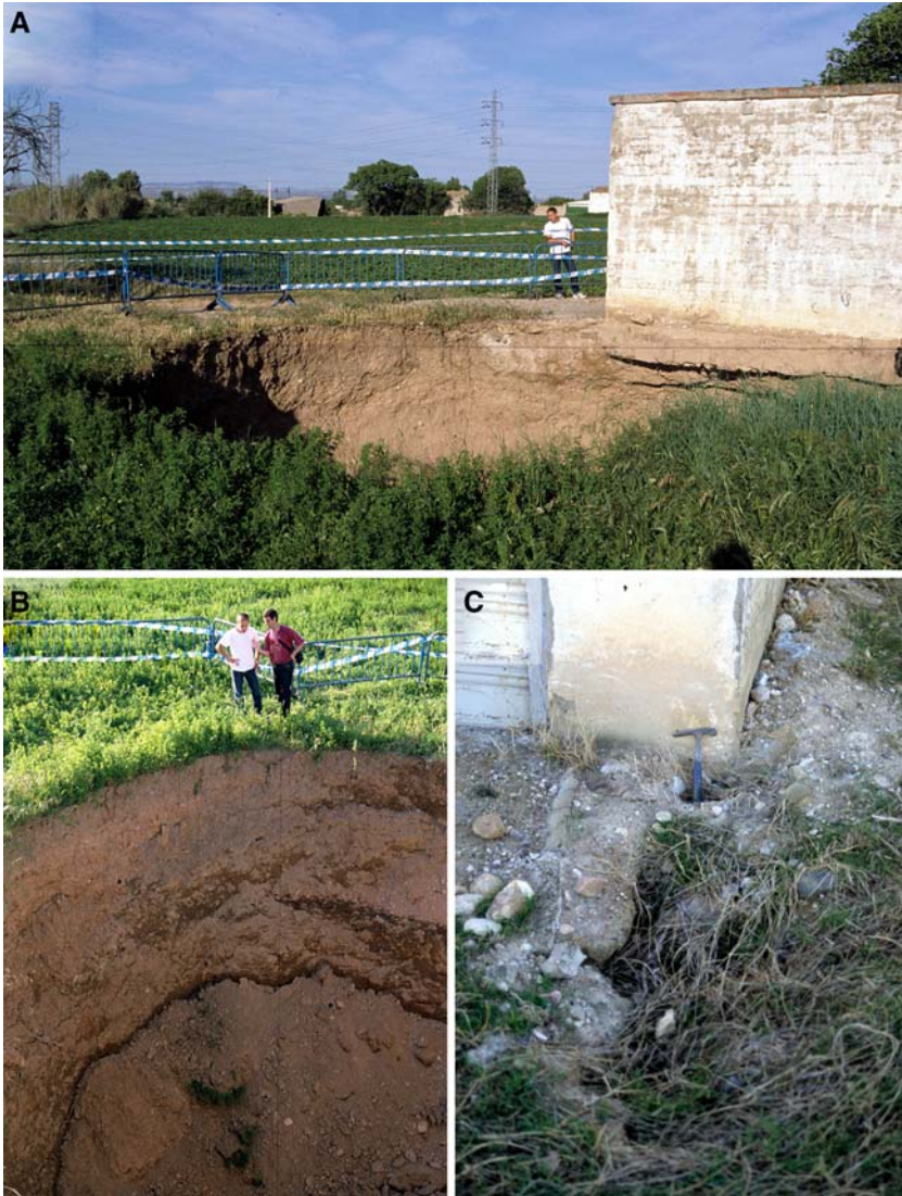
Fig. 7 (A) Sinkhole 4 formed on May 12, 2002; (B) close-up view of sinkhole 4. Photographs A and B were taken on 14 May 2002; (C) crack affecting the sinkhole fill in December 2004
