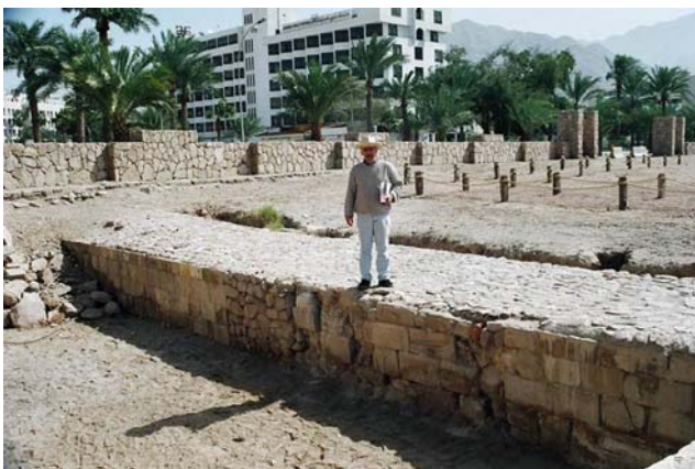
Fig. 8 Traces of poor quality repair in Ayla city wall to the NE from the city tower no. 4 (station no. 3)
