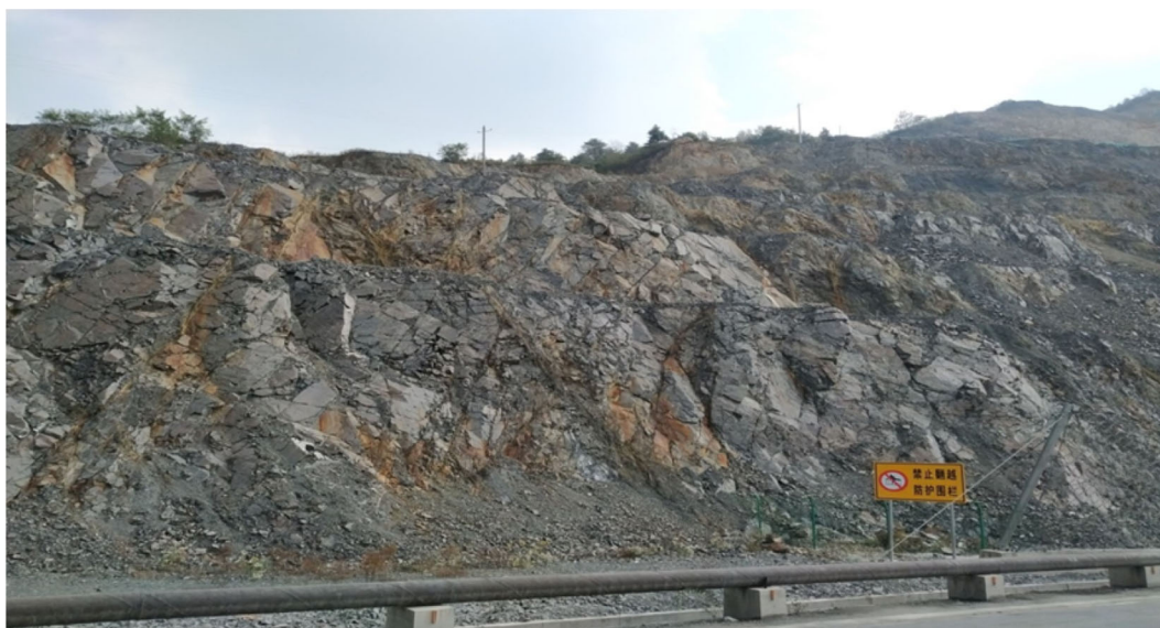
Figure 2. Jinduicheng north slope composed of multiple discontinuities and fault zones.
