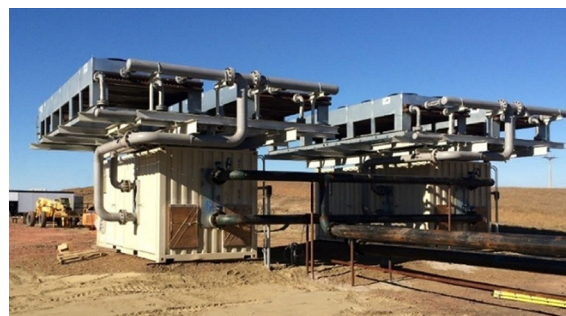
Figure 65. Photograph of a pair of binary electricity generating units producing electricity from hot produced water from North Dakota oil field. Image from: https://www.energy.gov/eere/success-stories/articles/eere-success-story-do-e-funded-project-first-permanent-facility-co .
