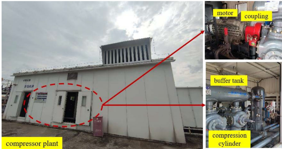
Fig. 18 Shale gas compressor site
