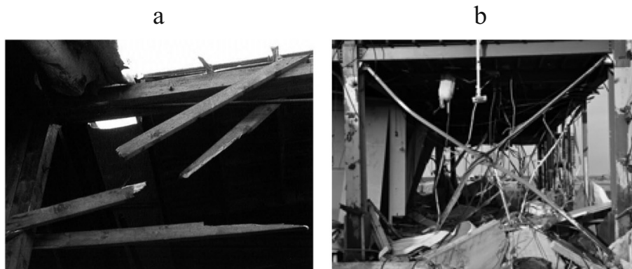
Fig. 5. Brittle failure of timber bracings (a) and ductile collapse of steel bracings (b).
