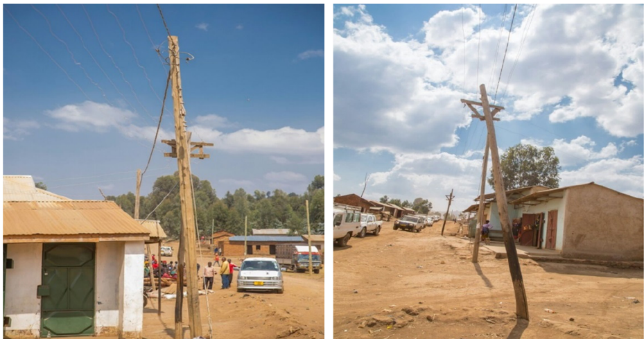
Fig. 3 Diesel engine powered rural mini-grid in Tanzania. Source: Authors' collected information in 2016
