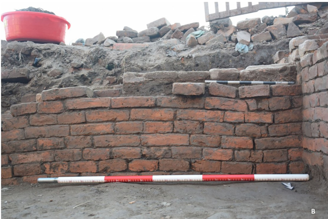
Fig. 10 Vertical cracks identified below a double saddle stone in the foundations of the Kasthamandap (a) and below a saddle stone in the foundations of the Gurujyu Sattal, Pashupati (b)
