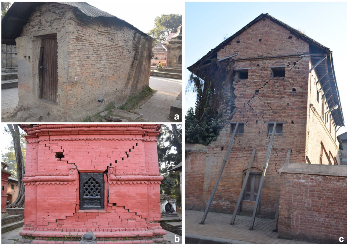
Fig. 3 Tilted wall at a structure at Mrigasthali in Pashupati (a); ‘X’ fracture through a brick built shrine at Mrigasthali in Pashupati (b); shear cracks through one of the walls within Bhaktapur Palace Complex (c)
