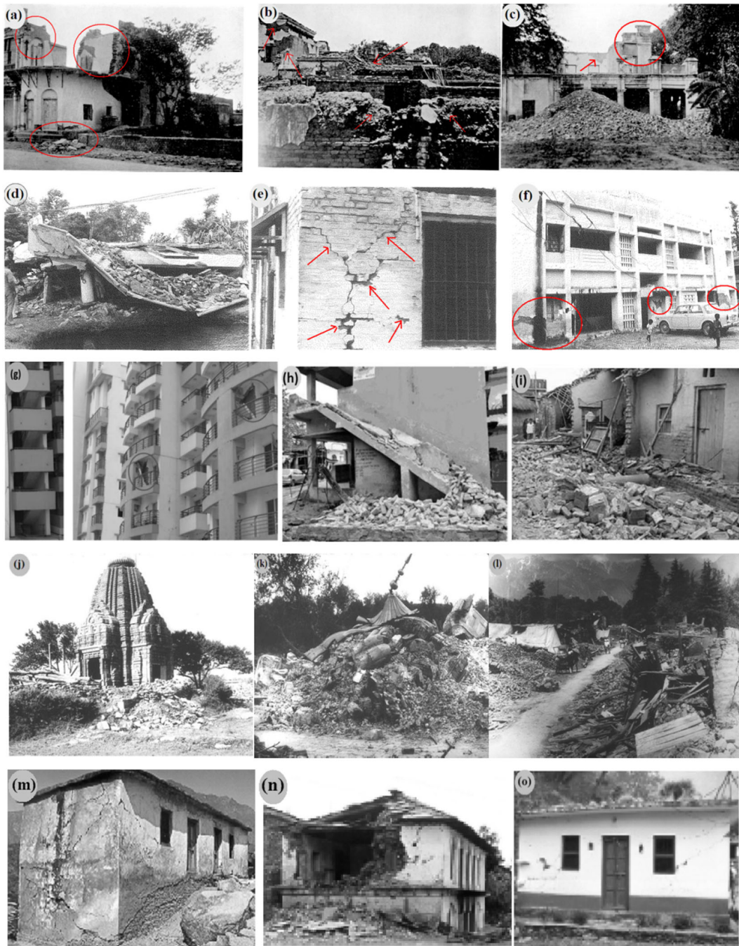
Fig. 3 Photographs of structural damage and building destruction due to near- and far-source moderate to large magnitude earthquakes viz. a–c 1934 Nepal-Bihar earthquake of M_w 8.1, d–f 1988 Bihar-Nepal earthquake of M_w 6.8, g–i 2015 Nepal earthquake of M_w 7.8, j–l 1905 Kangra earthquake of M_w 7.8, and m–o 1999
