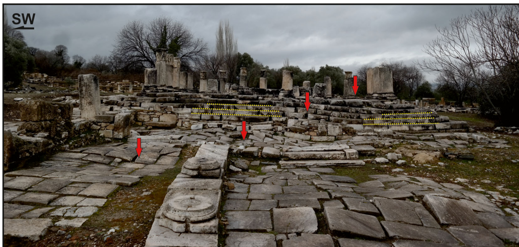
Fig. 10 Faulting along the temple and chapel. Red arrows show the fault (for location, see Fig. 7)
