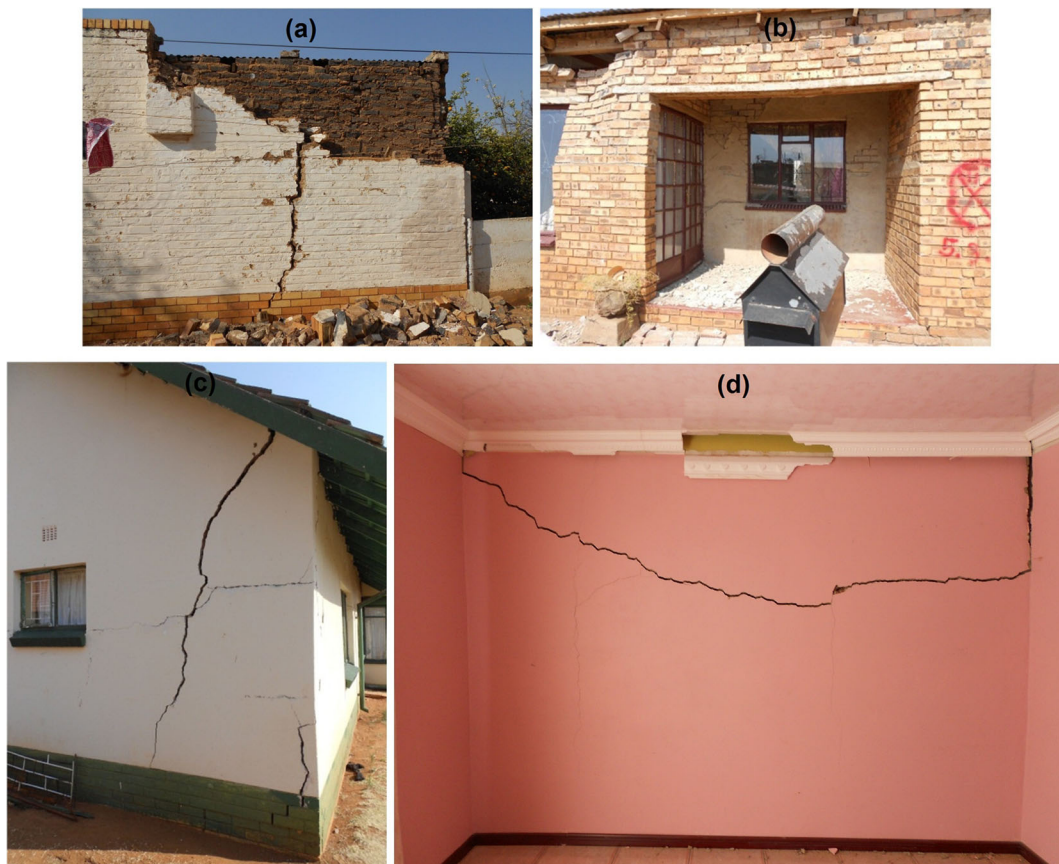
Fig. 3 Examples of observed damage to houses in the Orkney (a), Stilfontein (b, c) and Khuma (d) areas, which are located at epicentral distances of 15.8, 11.8 and 11.0 km, respectively. The photos of damage were taken by the CGS survey team during intensity damage survey
