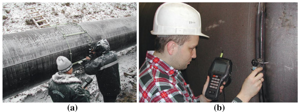
Fig. 43 Assessment of the material state and weld quality. a Execution of gas pipeline testing. b Weld inspection procedure [195] Copyright@2012, Welding in the World
