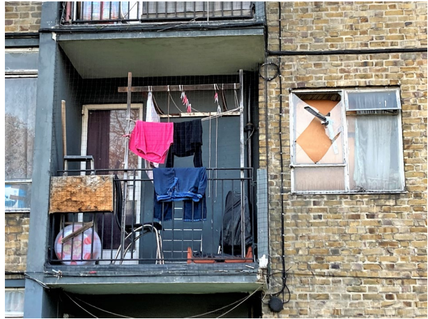
Fig. 4 Broken window in social housing flat at Clapham Park west, 2021 Photo: Paul Watt
