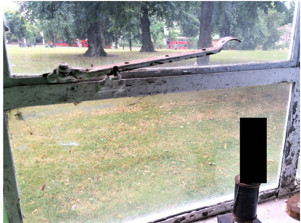
Fig. 5 Window frame from inside social housing flat at Clapham Park west, 2016 Photo: Paul Watt
