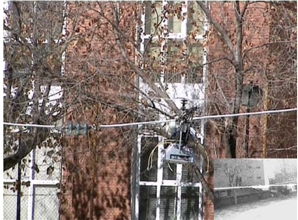
Fig. 16 Power line and Isolator detection using the UAV vision system
