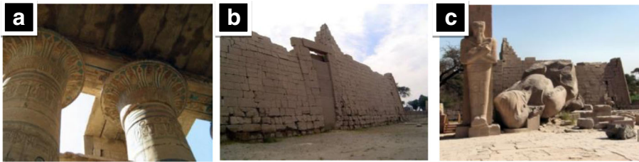
Fig. 9 The archaeological deteriorations as a result of the environmental risks (a–c) (Ramesseum temple)
