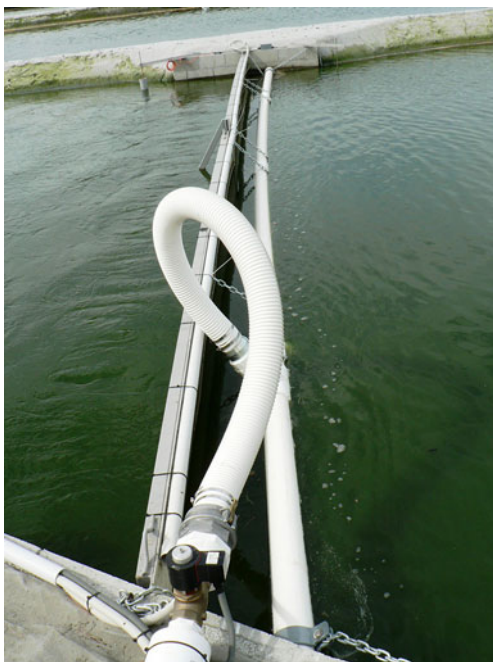
Fig. 5 Photograph of the Christchurch demonstration HRAP CO 2 addition sump
