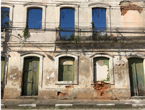
Fig. 2. Current situation on the side of the building. Credit: Wagner Magalhães – July 2018
