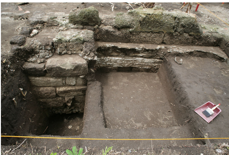
Fig. 13 The column base foundation along the western portion of the north wall of Structure B measuring 140 cm thick compared to the foundation of the wall which is 50–58 cm thick
