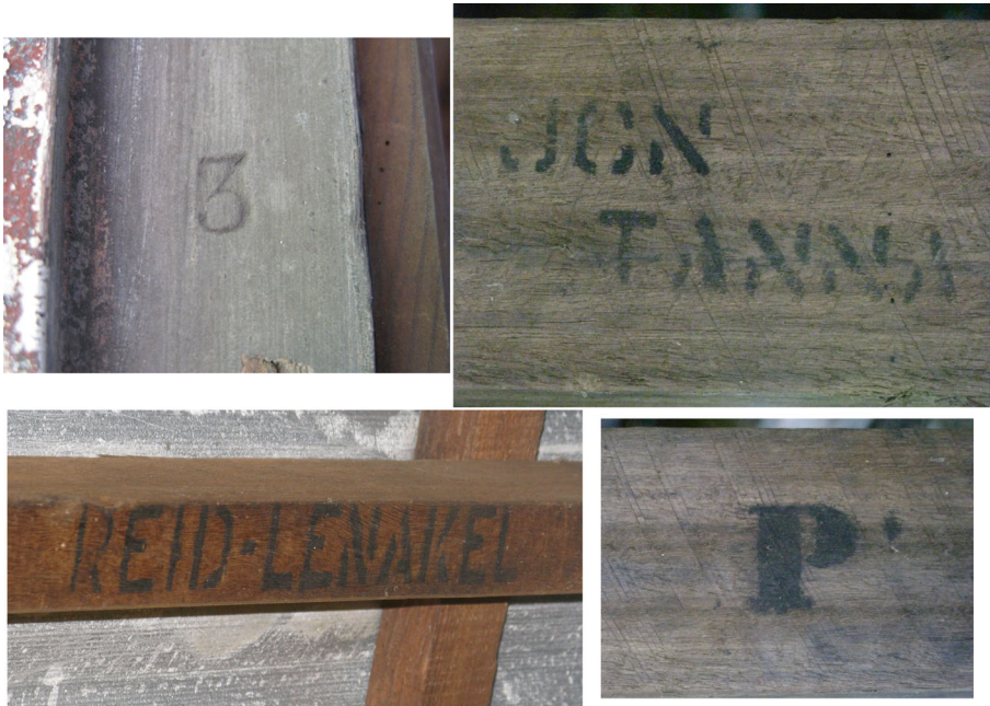
Fig. 7 Consignment and assembly marks on Lenakel Mission buildings, clockwise from top left: “3” assembly mark, Lenakel Church; “JCN TANNA” consignment mark (note also machine saw marks), Lenakel Church; “P” possible consignment or assembly mark, Lenakel Church; “REID-LENAKEL” consignment mark, from later nuns’ house
