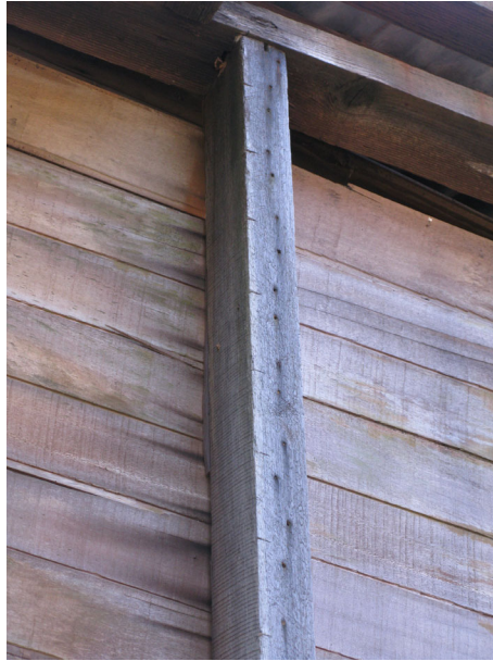
Fig. 10 Example of laying-out marks on vertical studs to assist placement of horizontal wall boards
