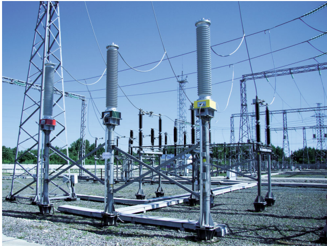
Fig. 5. General view of the HVPC installed at the 220 kV switchyard during the PO at the 220 kV substation of FSK EÉS PJSC.
