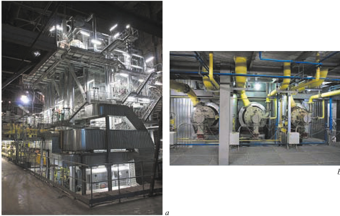
Fig. 3. Boiler unit No. 4 installed at the VKG ENERGIA OÜ electric power station in Kohtla-Järve (Estonia): a , general view; b , burners for shale processing gas combustion.
