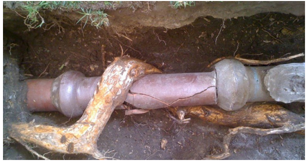
Fig. 3 Roots growing around a pipe
