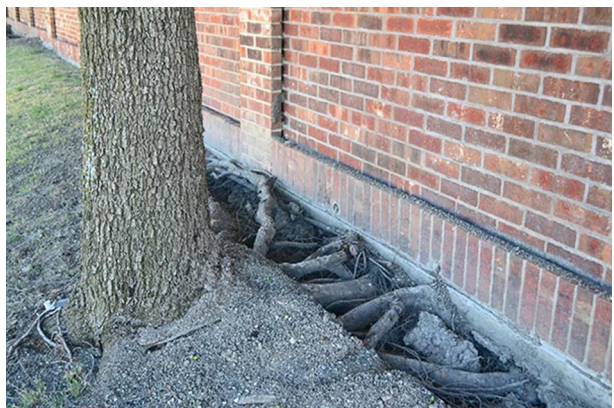
Fig. 2 Tree roots growing under foundations
