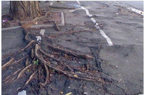
Fig. 4 Damages to road pavement due to tree roots
