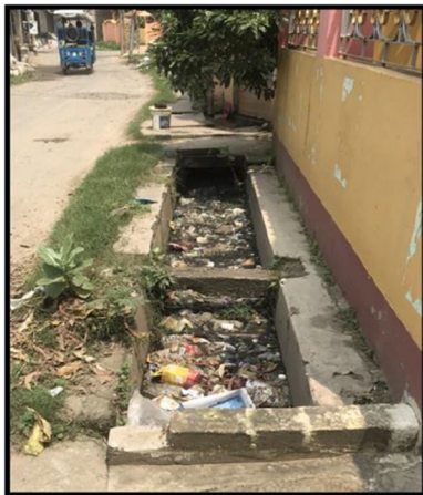
Image.6 The drain is filled with trashes Source: Field Survey, April, 2023 (Fig. 11)
