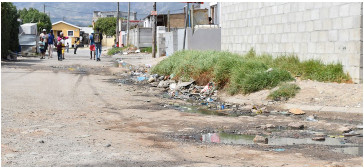
Fig. 15 Sewage and litter collecting along the street after the rains. (Author's own)
