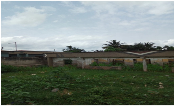
Fig. 9 Abandoned buildings situated in a wetland, Atonso S-line
