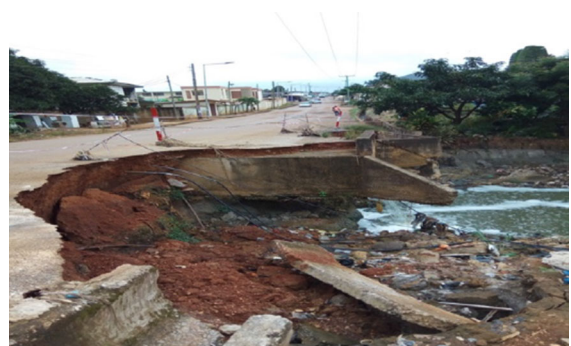
Fig. 11 Stream erosion-induced Collapse Bridge (Kwadaso)
