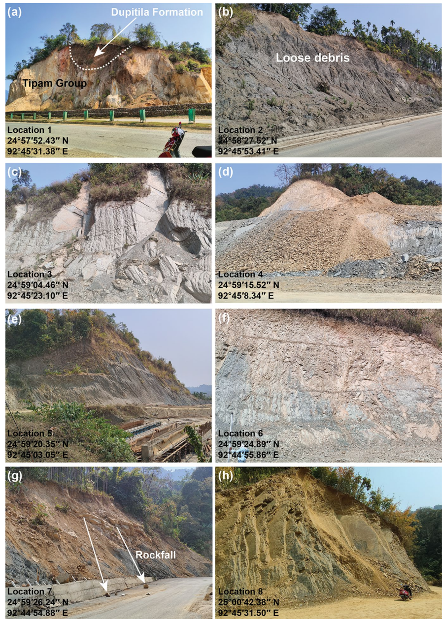
Fig. 3 Field photographs depicting present-day rock mass condition along the Silchar-Haflong NH, a Polymictic conglomerate of Dupitila Formation at the top and massive medium-grained Tipam sandstone at the bottom, b Loose and weathered debris material, c Bhuban sandstone with daylight bedding planes, d Recently exposed cut slope in Bhuban sandstone, e very weak and friable Bhuban shale with bedding plane dipping towards the slope, f recently excavated road cut slope in Bhuban sandstone, g view of rockfall (sandstone blocks), h thinly bedded hard massive Barail sandstone dipping towards towards slope face
