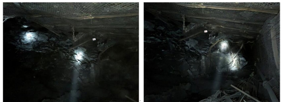
Fig. 15 Roof strata caving in the goaf
