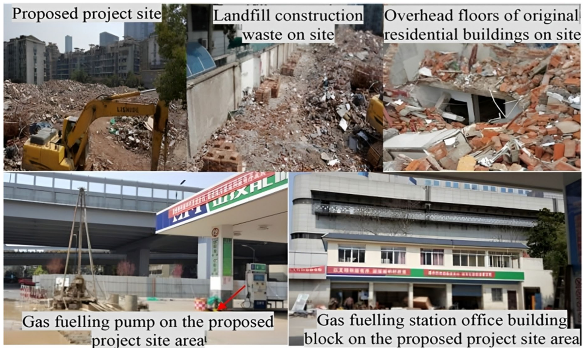
Fig. 2 Triumph Unit construction site showing the environmental condition of the site topography and landforms prior to commencement of basement excavation
