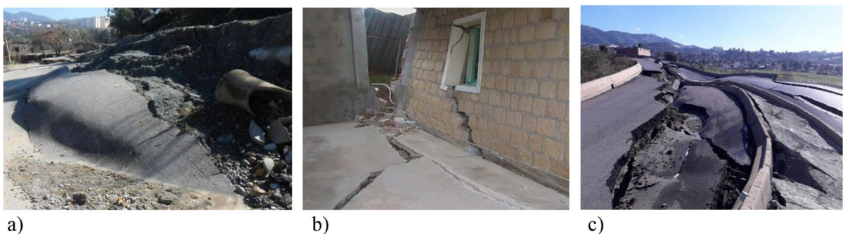
Fig. 1 Various damages caused by landslide in Azazga region on a a sewerage system in March 2012, b a house in March 2014, c a road with the appearance of subsidence in January 2019
