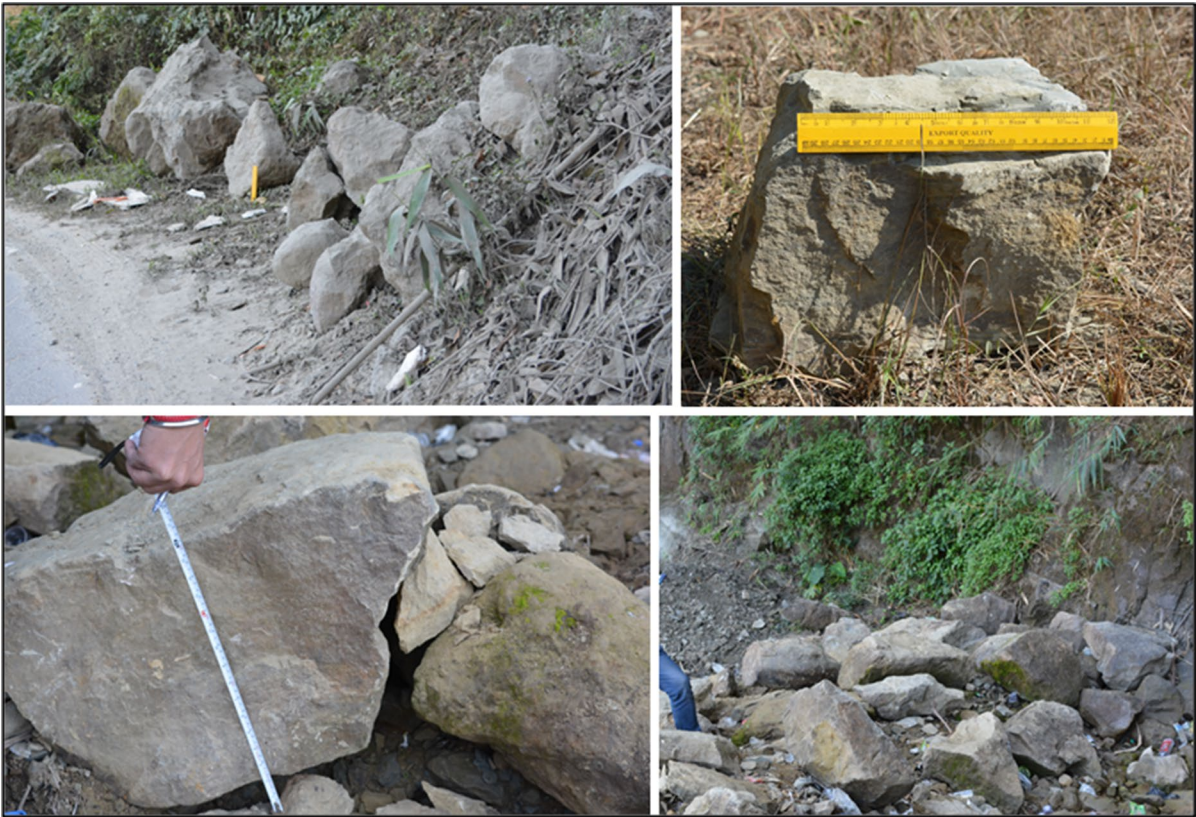
Fig. 4 Field photographs showing falling rock blocks along NH-44A, Aizawl
