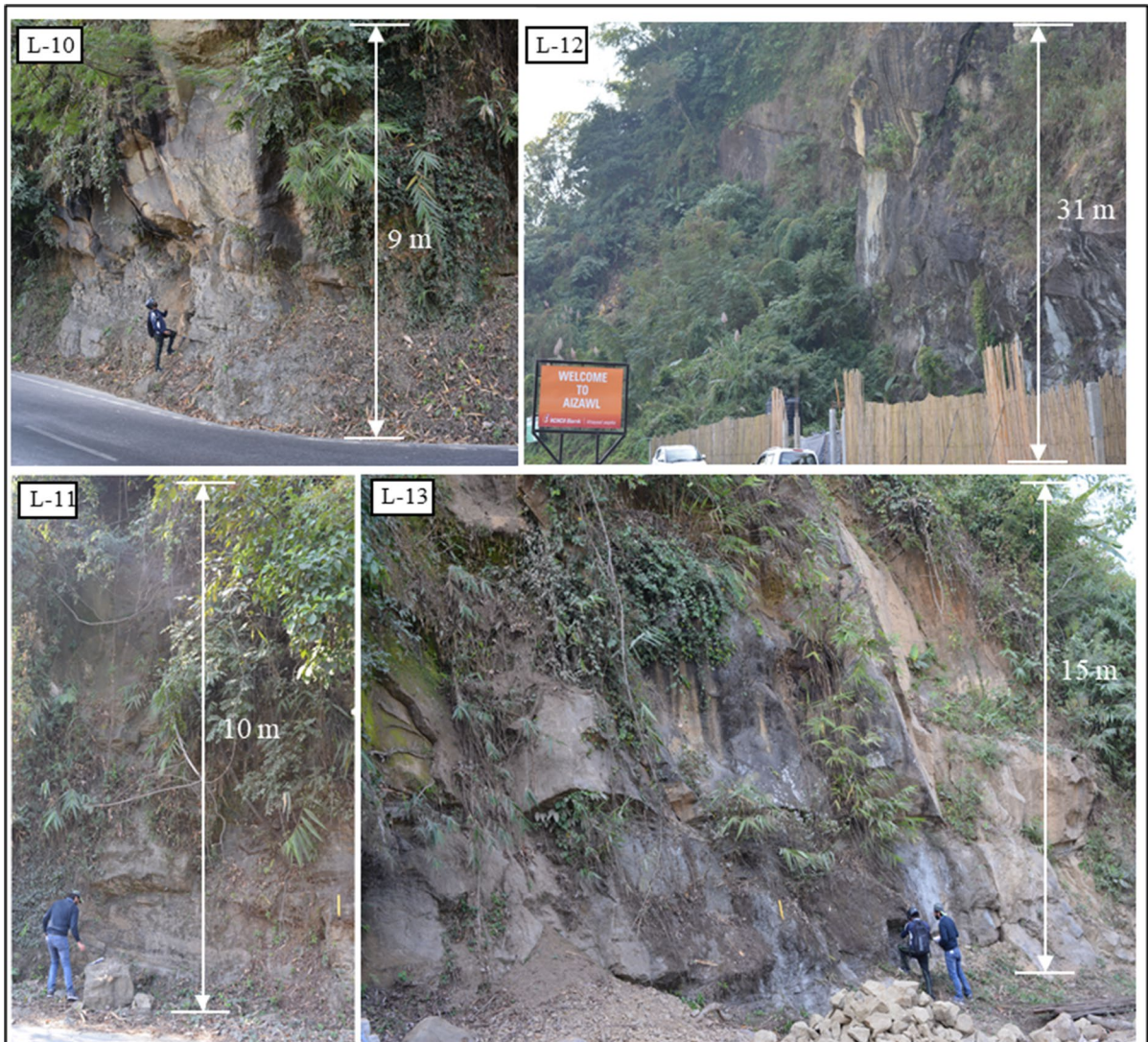
Fig. 3 Field photographs showing road cuts (L-10–L-13) along NH-44A, Aizawl
