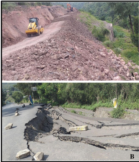
Fig. 9 The figures, show maintenance of the A roadside slide, and B Road slides
