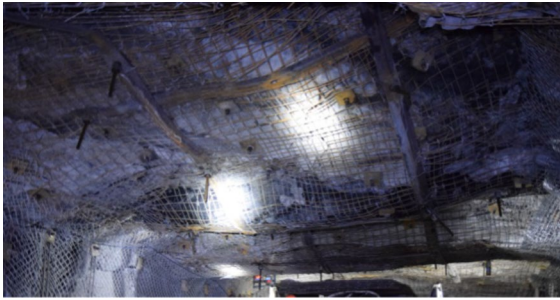
Fig. 1 Deep buried high stress and large deformation roadway (reproduced from literature Yang et al. (2020))
