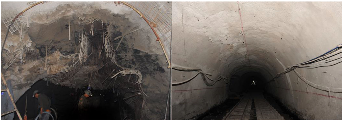
Fig. 5 Comparison of roof deformation before and after – 980 m roadway support
