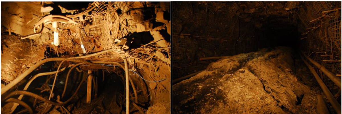
Fig. 1 Roadway damage map
