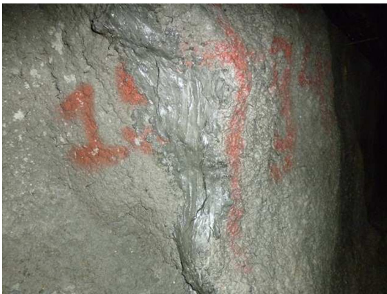
Fig. 13 Ring crack, several shotcrete cracks observed along the crown and both walls with opening up to 1.50 cm at chainage 15 + 937
