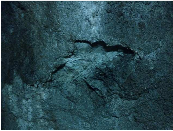
Fig. 12 Spalling, shotcrete fall from right wall along shear band, area up 1sqm at chainage 16 + 823
