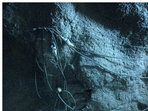
Fig. 11 Lining crack, up to 7 mm at chainage 18 + 239
