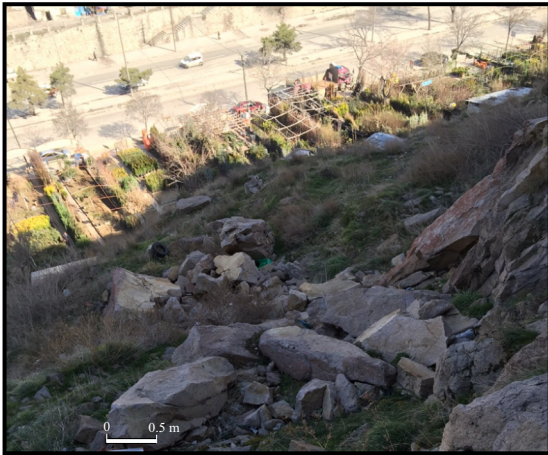
Fig. 3 Fallen blocks seen near the floral shops and the road
