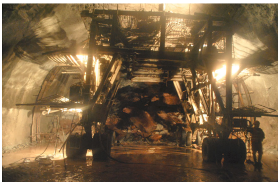
Fig. 12 Actual situation of the collapse in the tunnel (Li et al. 2014)
