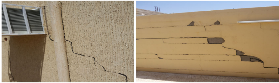
Fig. 1 Structural damage due to collapsible soils below the foundations in Najran area (Rouaiguia and Dahim 2016)
